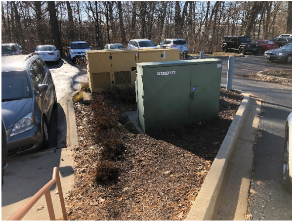
Photo 1: Existing generator and Utility Transformer.
